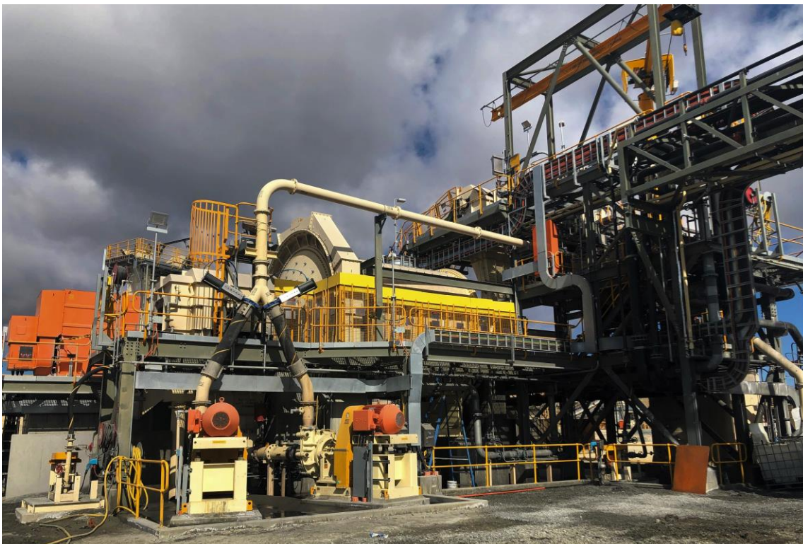
Figure 1 Ball Mill during the underground crushing and grinding circuit commissioning campaign.
