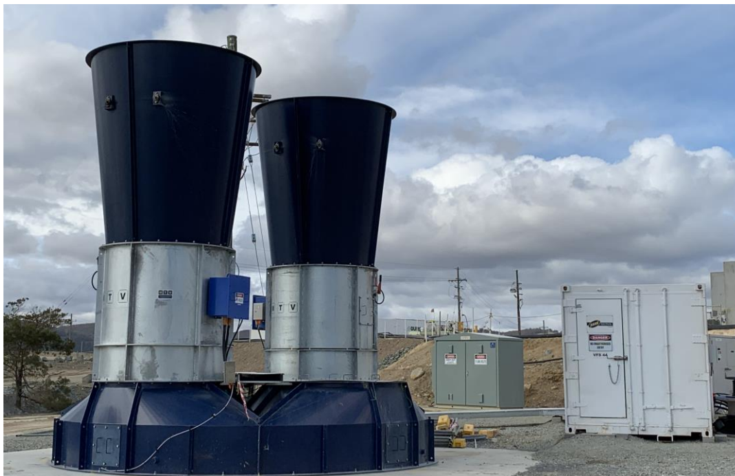
Figure 4 New vent fans installed for underground and operational.
