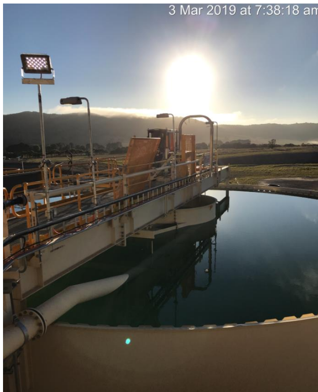
Figure 1 Tailings thickener undergoing wet commissioning
