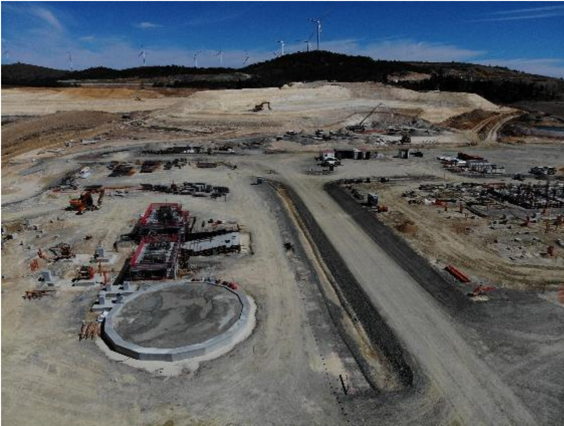
Figure 3: Reclamation area (left), flotation area (right) and concrete pour at the primary crusher (rear).
